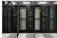
The University of Texas's Stampede supercomputer, on which the 200-terabyte maths proof was solved. Credit: University of Texas
